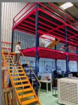
Industrial Mezzanine Floor
